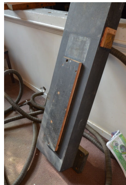
Figure 3 Swell low-pressure trunking with a roughly fitted blanking plate where concussion bellows would have fitted (photo John Page)
